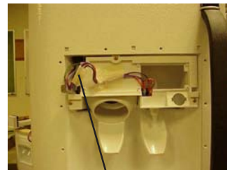
Connector from door harness to actuator switches
