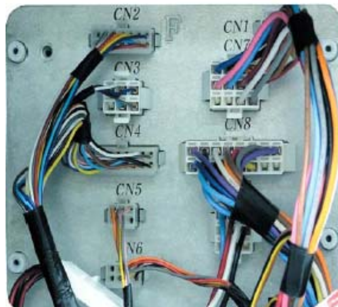
Terminal Block Panel with Cover Removed
