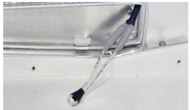
Drain heater removed from drain
