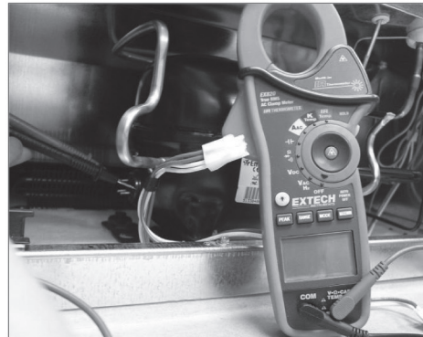
Measuring compressor motor resistance
